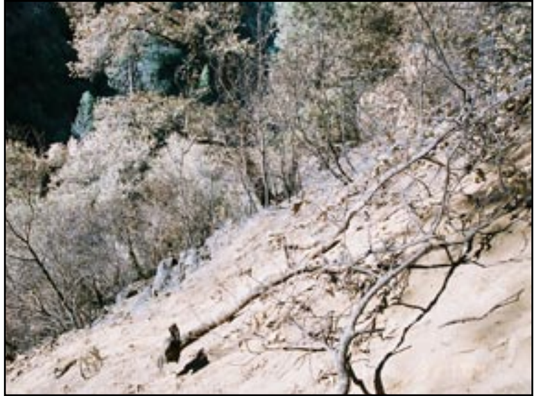
Fireline construction area. Lumsden Road is to right of photo. Rock outcropping is in center of photo.
